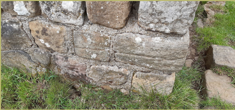
Section of the wall at Milecastle 39 showing outer sandstone blocks and lime mortar
